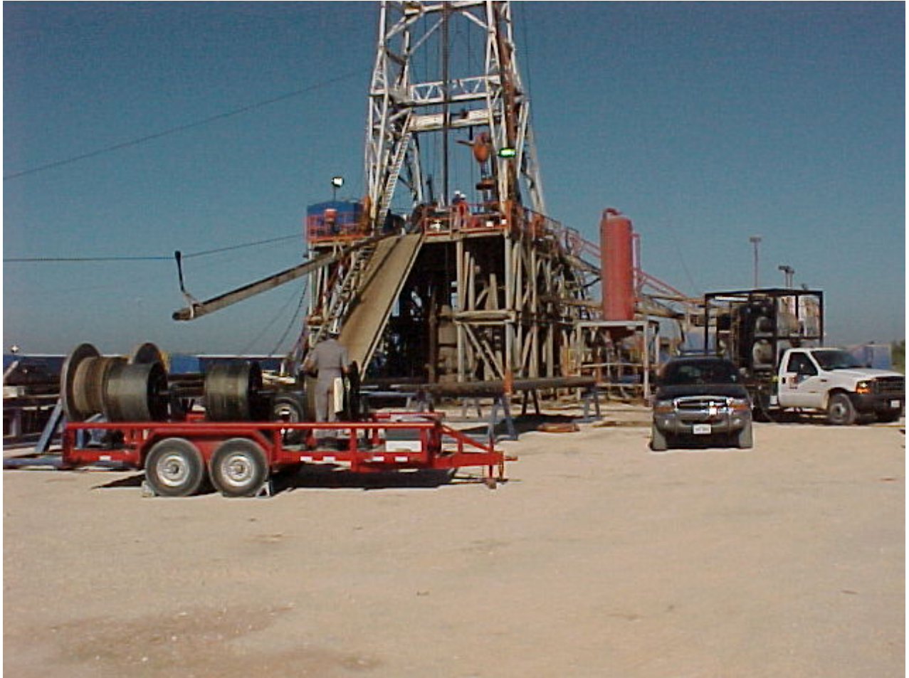
Figure 7.1 – CPU and Cable Trailer at Mestena #E-25
