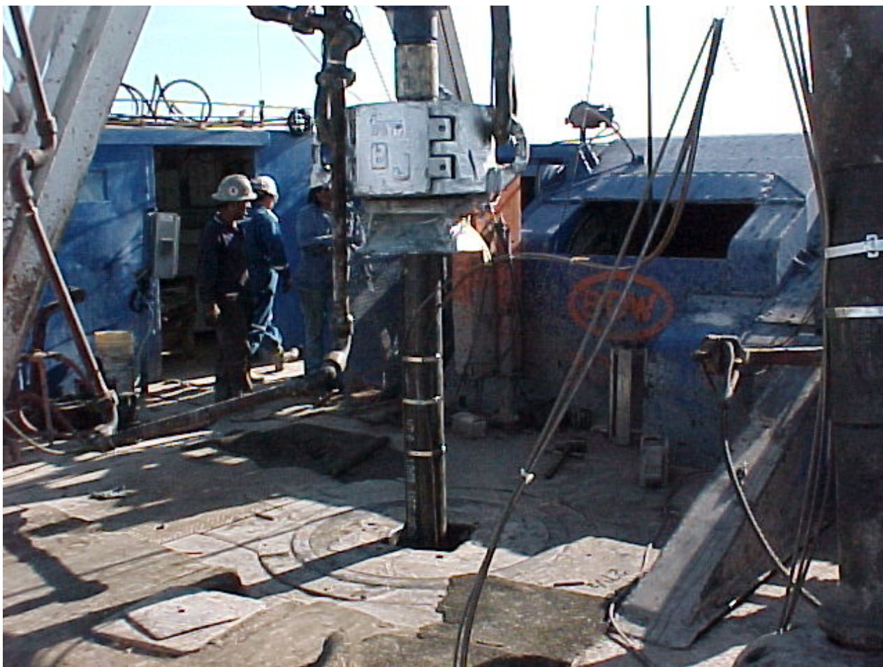
Figure 7.4 – Cables Banded Below the Elevator
